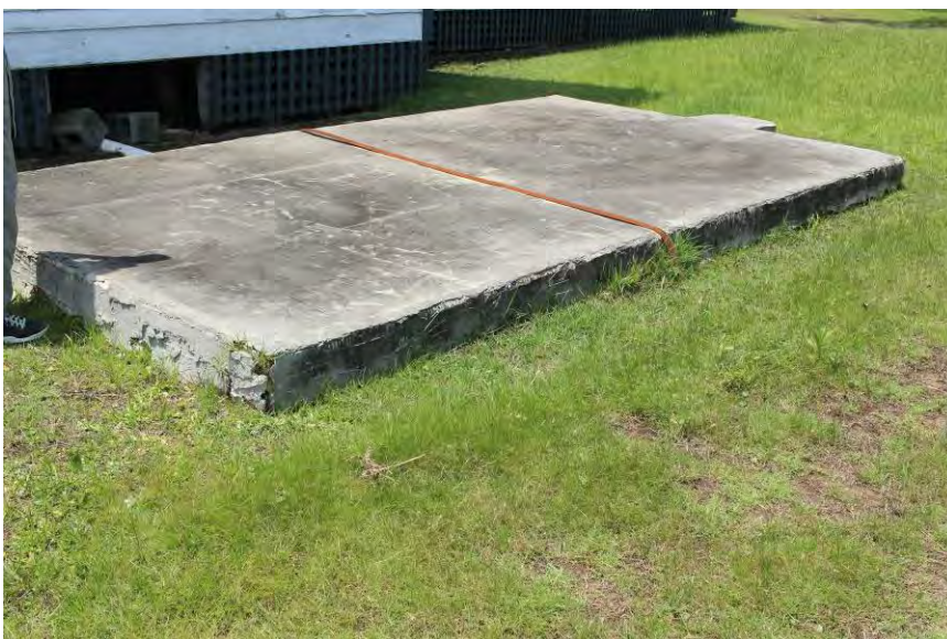
FIGURE 139. Rectangular concrete slab north of the Theodore and Annie Salter House that covers a septic tank.
