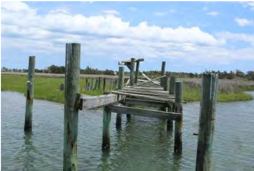
FIGURE 90. View of the damaged dock and boardwalk behind the Styron and Bragg House.
