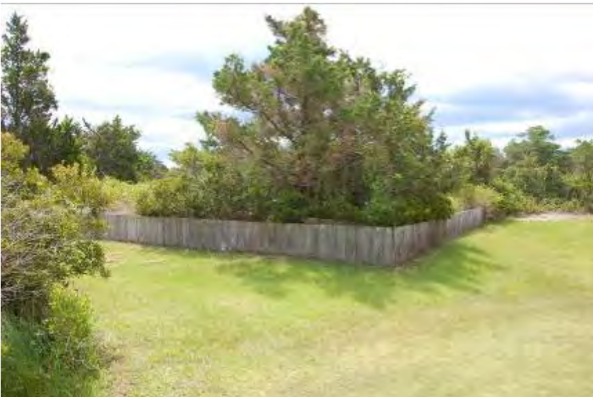
FIGURE 135. Septic leach field with wood surround, located southwest of the Life-Saving Station.
