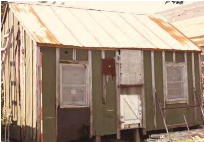
FIGURE 74. The north facade of the summer kitchen east of the Carl Dixon House, circa 1979.
